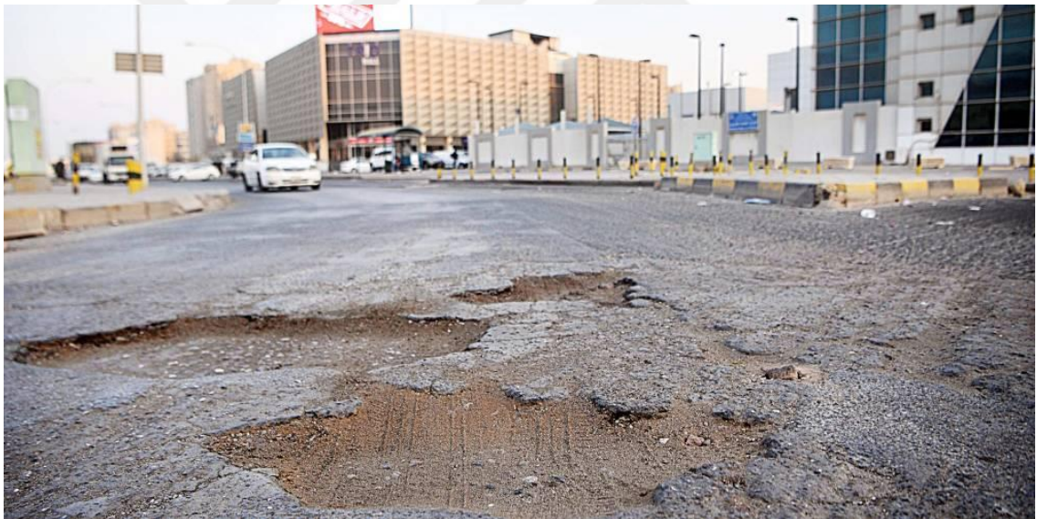
Figure 1.1: Poor Road Maintenance
