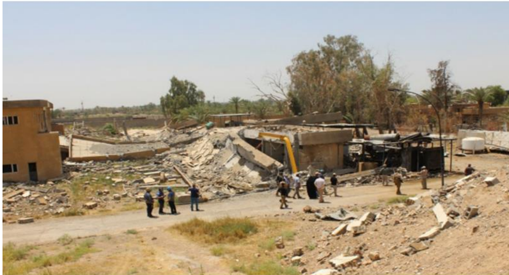
Figure 3.1: WTP 2 (Al-Azrakiyah Water Treatment Plant) Before Rehabilitation in August 2016
