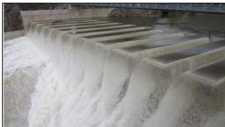
Figure 2.7: View of the PKW spillway of Malarce Dam in France during spillage.
