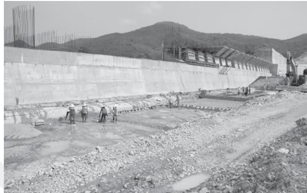
Figure 2.16: Treating the downstream of PKW to protect against erosion, (Van Phong Dam) in Vietnam.
