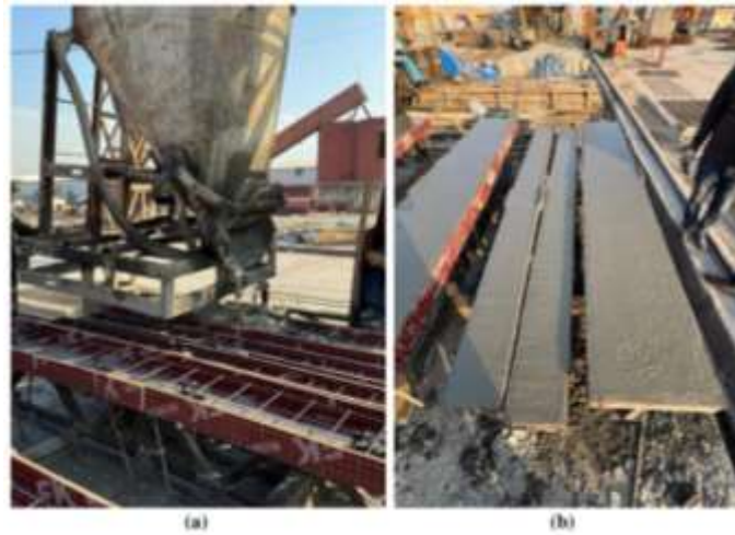
Figure 4.32: Steps of Concrete Pouring the Main Truss Girder (SCTG) and (DCTG). (a) Poring the Concrete Mix Stage, (b) Final Step of the top and Bottom Concrete
