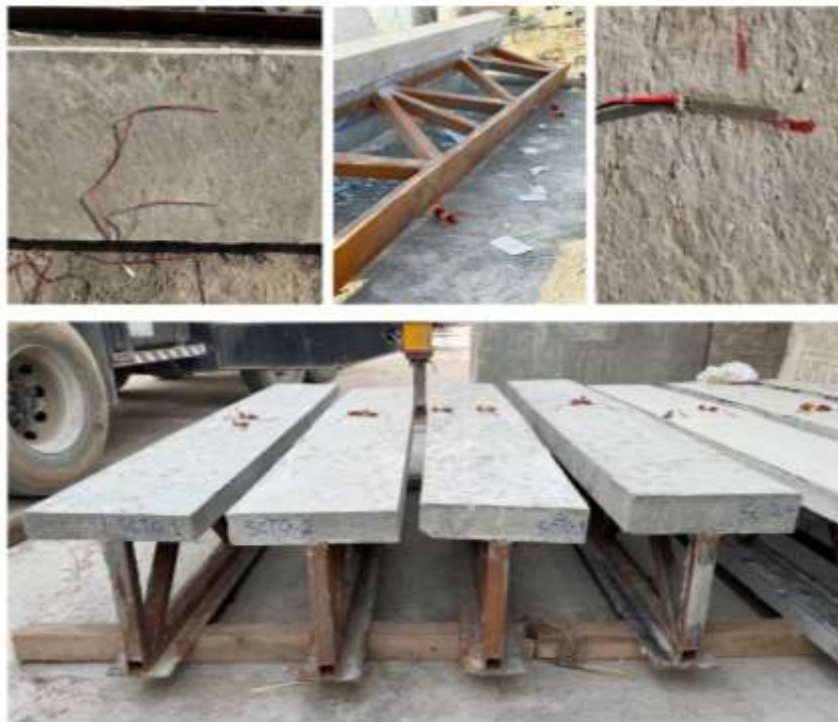
Figure 4.37: Position of the Strain Gauges for Category One Specimens (SCTG). (a) Strain Gauge Location Drawing sheet for the (SCTG), (b) Site Installation of the Strain Gauge for the (SCTG)
