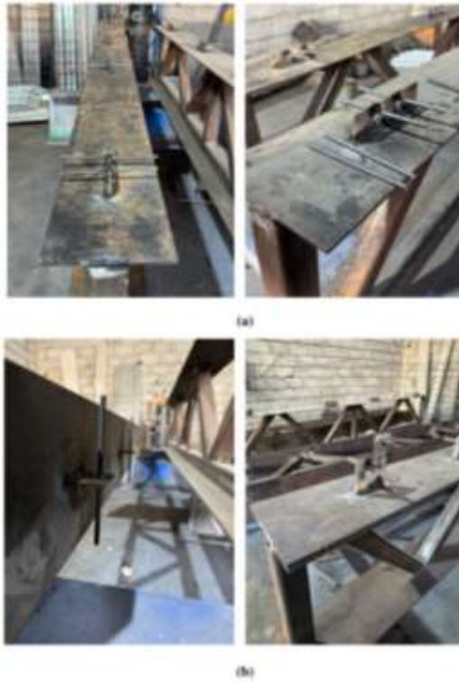
Figure 4.23: Holes Steel Plate Bars Instillation of Category Two Specimens (DCTG). (a) Top Holes Bars of Perfobond Leiste Shear Connector Installation, (b) Bottom Holes Bars Perfobond Leiste Shear Connector Installation
