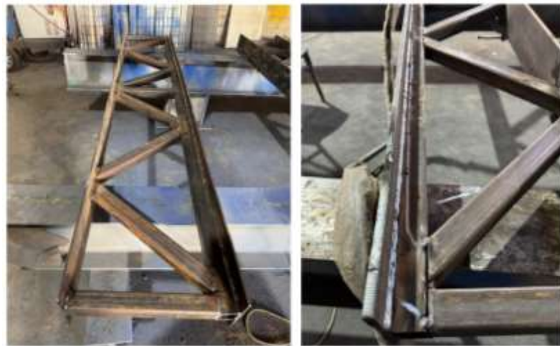
Figure 4.19: Main Structure Body Manufacturing of Category (SCTG). (a) Side View of the Truss Girder (Steel Plate With Vertical & Diagonal HSS), (b) Side View of the Truss Girder (Welding Stage of the Bottom HSS)
