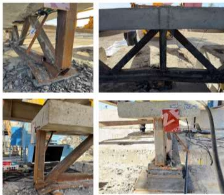
Figure 6.7: Failure Mode of the SCTG-4
