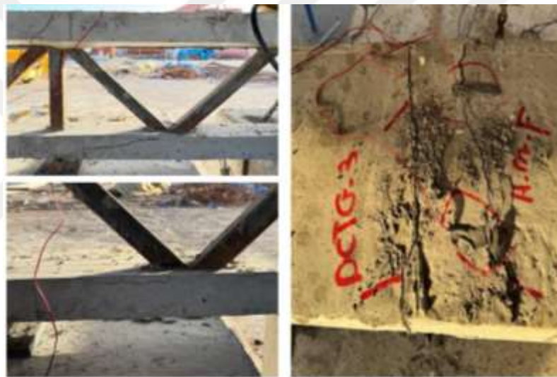
Figure 6.34: Initial and Ultimate Cracks Pattern of the DCTG-3
