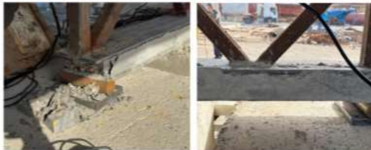
Figure 6.31: Failure Mode of the DCTG-4
