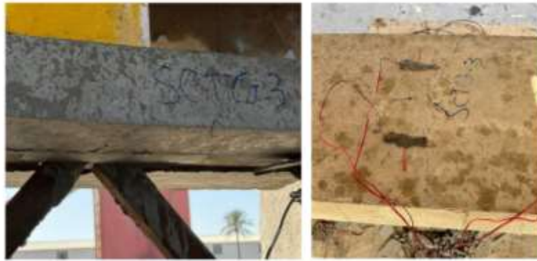
Figure 6.10: Crack Pattern of the SCTG-3
