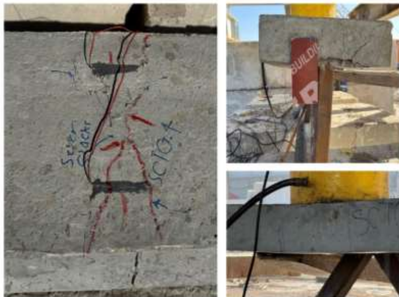
Figure 6.11: Crack Pattern of the SCTG-4
