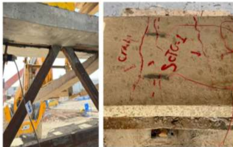
Figure 6.8: Crack Pattern of the SCTG-1
