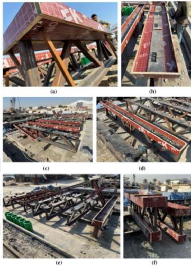
Figure 4.28: Main Eight Specimens' Wooden Molds site Installation. (a) Supports the Top Mold With Steel Bars By Welding, (b) Top Mold Installation, (c) Sliding the Molds to the Steel Girder, (d) Bottom Mold Installation for (DCTG), (e) Bottom and Top Mold Installation, (f) Top Mold Installation for (DCTG)
