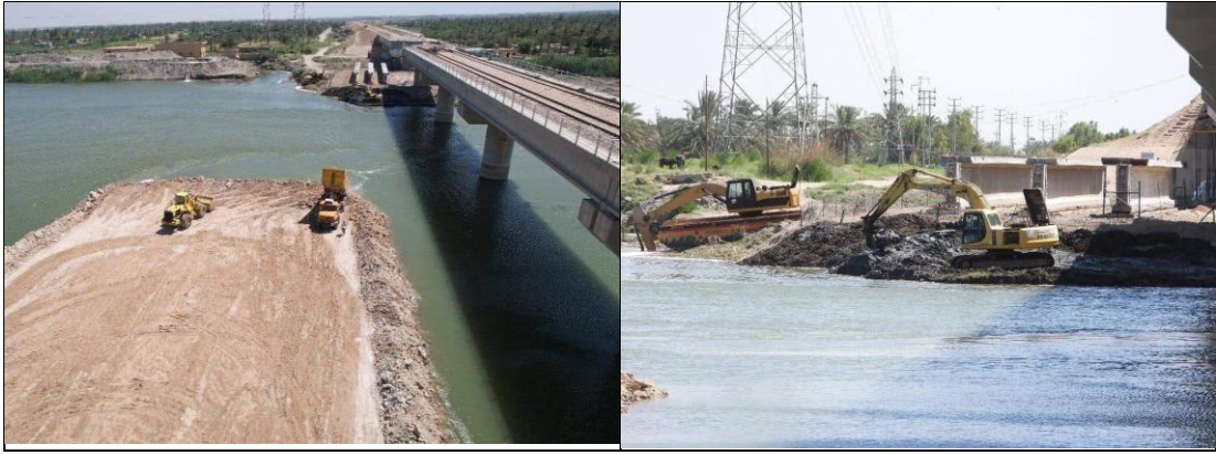
Figure 3.4: Fallujah's Fourth Bridge in Anbar (RW)
