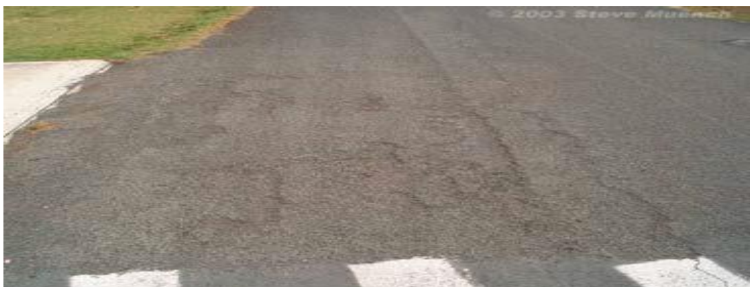
Figure 2.13: Raveling & Weathering Problem
