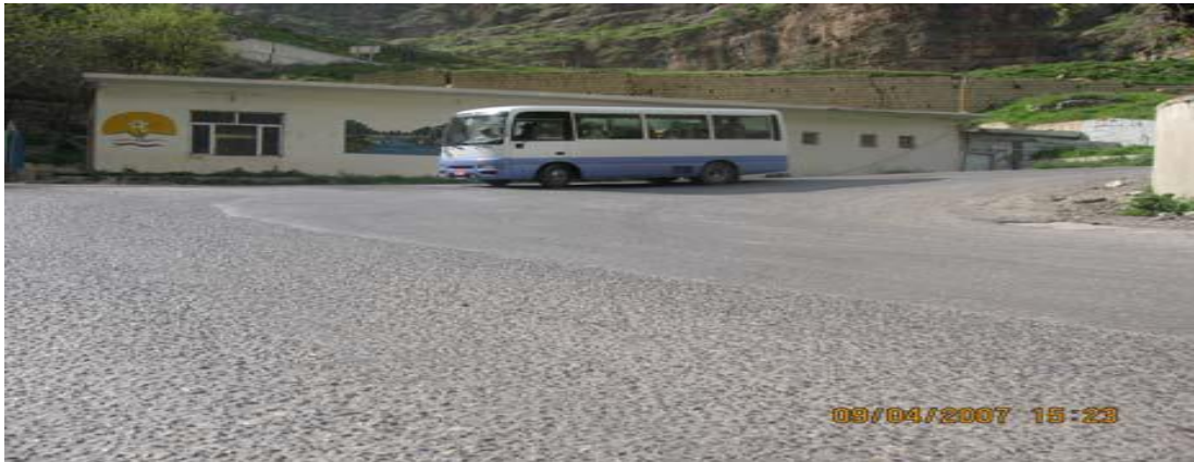
Figure 2.14: Polished Aggregate Problem
