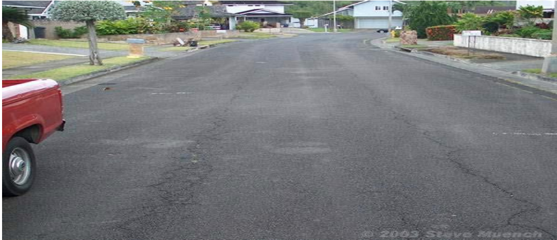
Figure 2.2: Longitudinal & Transverse Cracks
