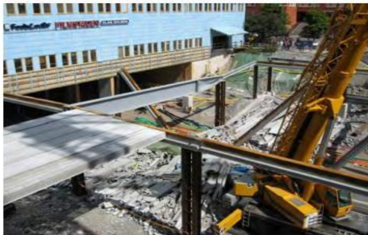
Figure 2.4: Same View as in Figure (2.3), After Collapse
